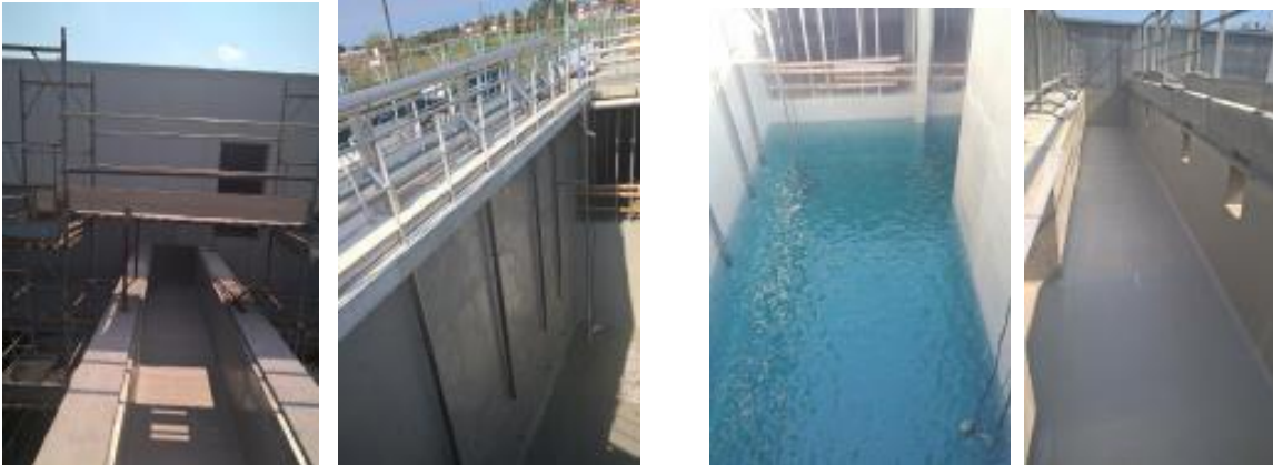
Our reference in Cittadella (Italy): Drinking Water Treatment Plant
