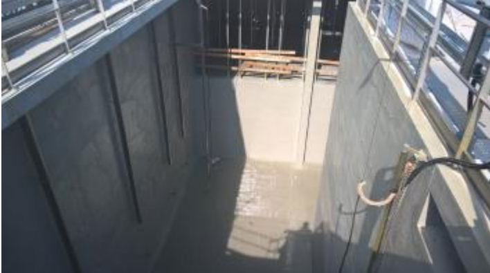
Our reference in Cittadella (Italy): Waste Water Treatment Plant
